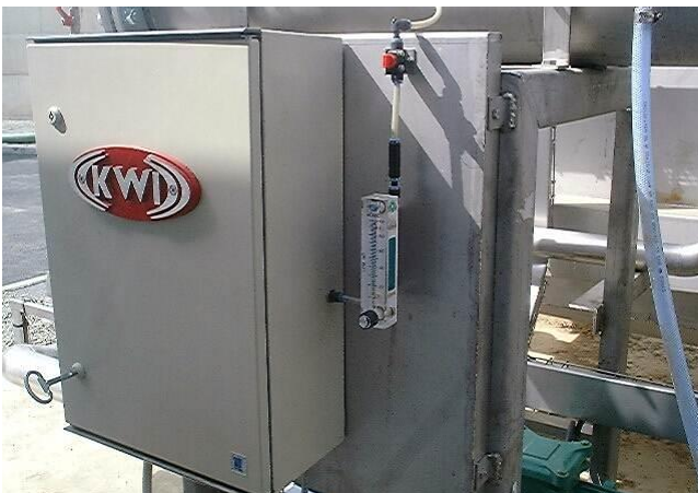
Air panel in a case protection with its display rotameter and regulation
