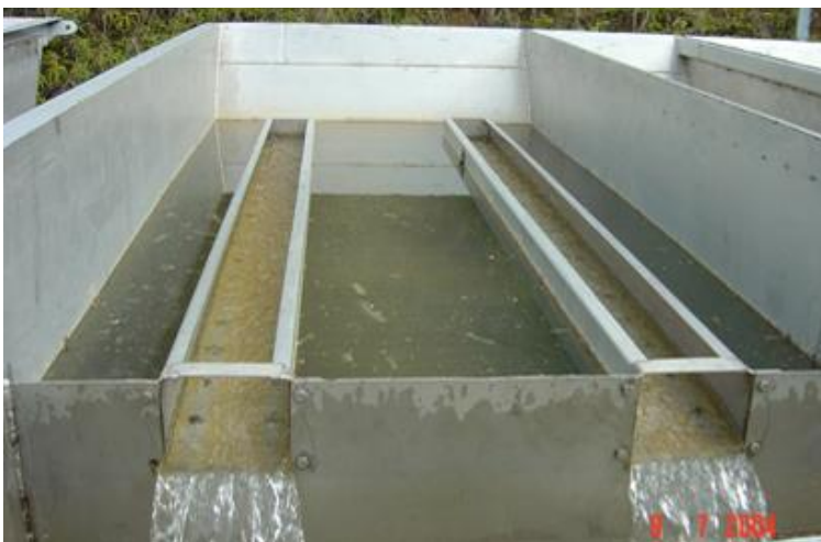
Clarified water overflow from lamella settler
