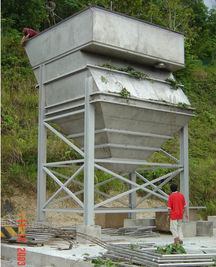
1 st Lamella settler in position
