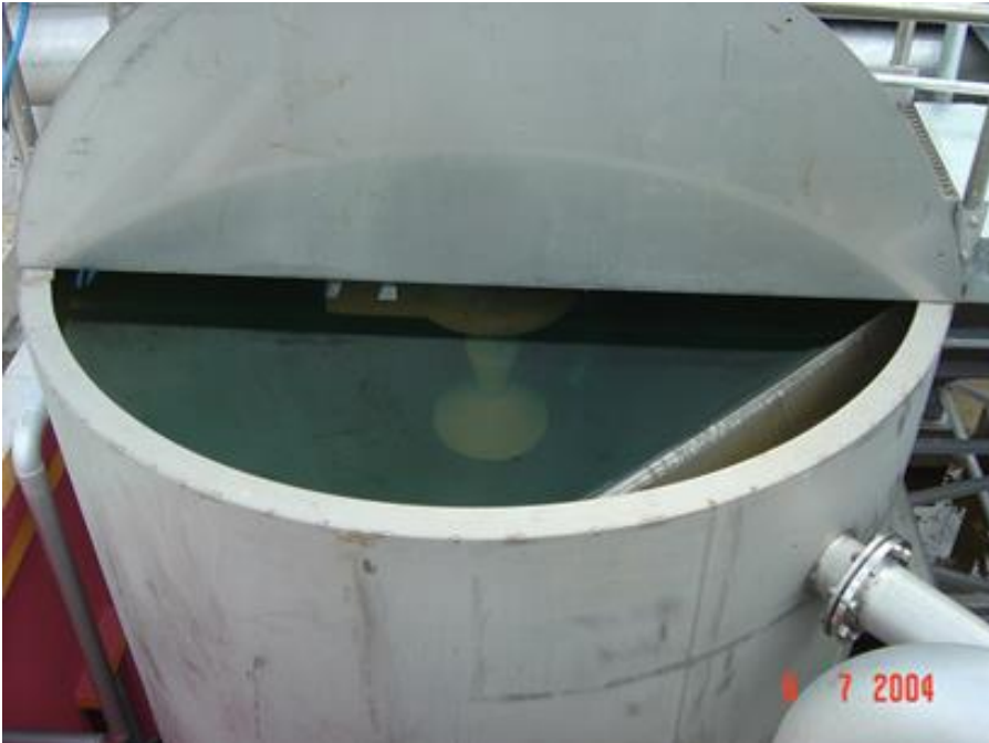
Filtered water overflow KSF.
